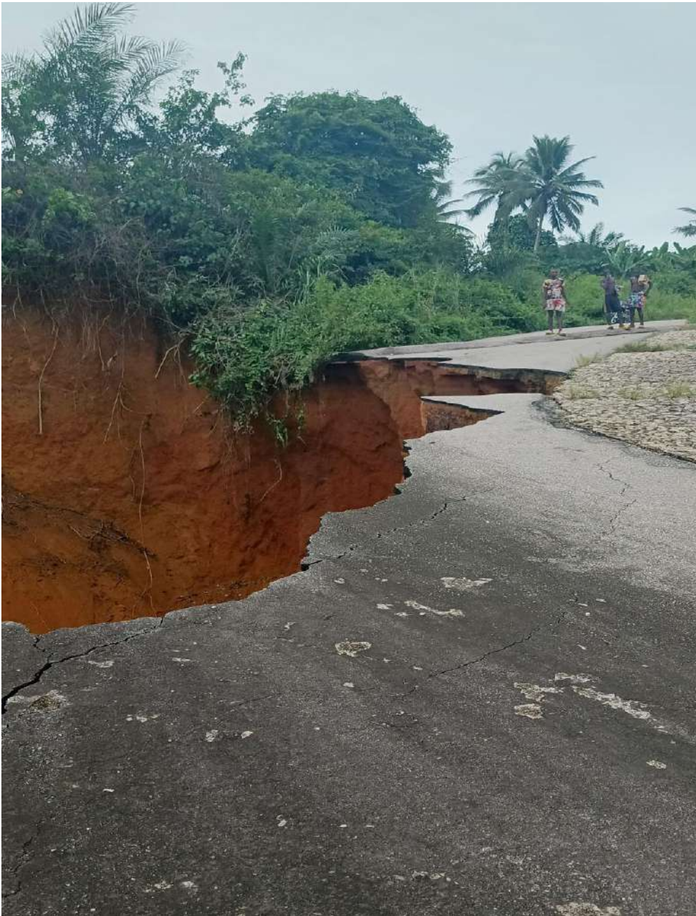
Picture Showing Gully Erosion caused by Heavy Rainfall in Esuk Mba
