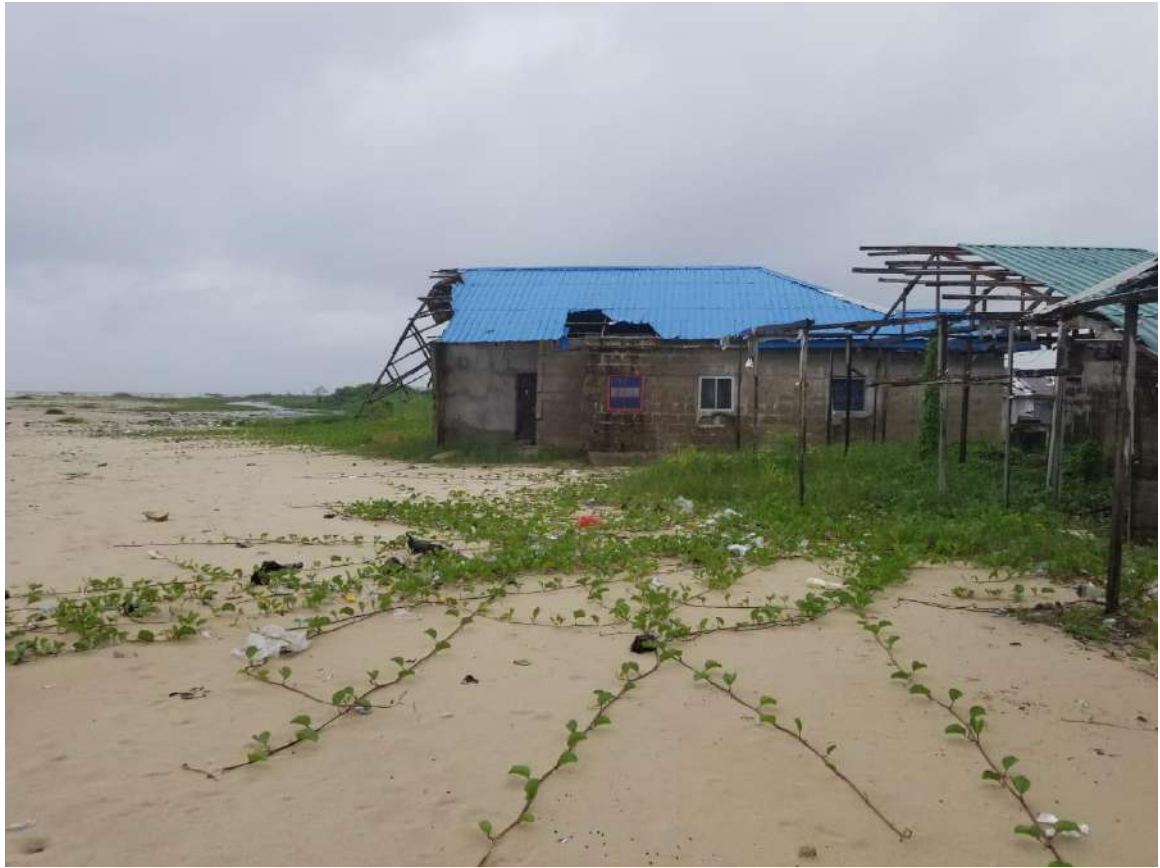
Picture Showing How Rise in Sea Level and Sea Surge Washed Away Residential Houses in Inua Eyet Ikot, Ibeno LGA.
