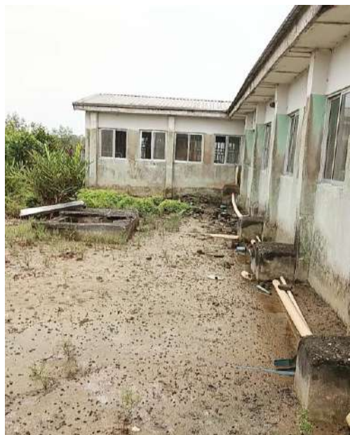
Flood Ravaging Health Centre in Agbakabiriyai Nembe Kingdom
